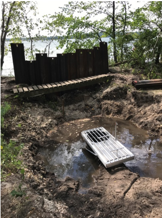
Slide gate assembly bolted to weir tee. Top of riser pipe set at 867.60'
