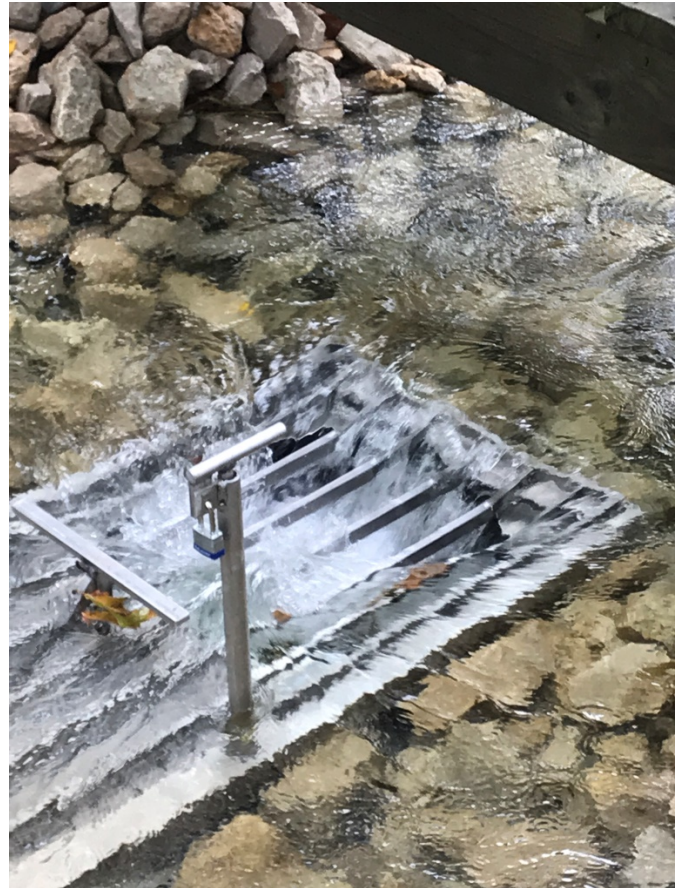
Slide gate lock and level indicator
