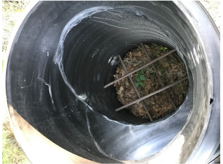
Rebar rods to stabilize structure. Concrete added in bottom of tee up to the side discharge.
