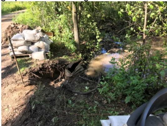
Original exit pipe bent to prevent water backup.
